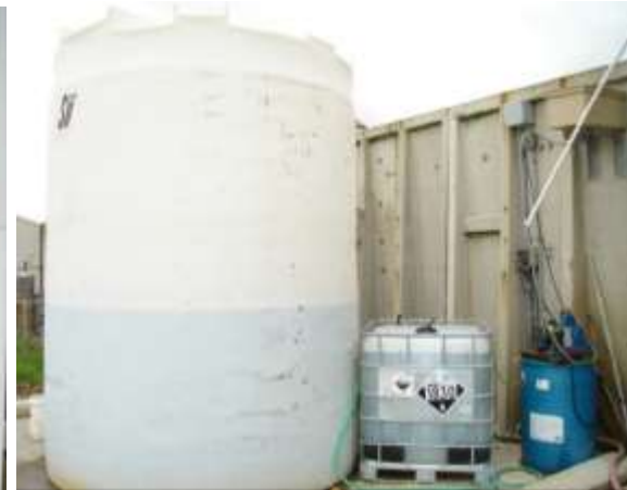
Ammonium Sulfate Tank
