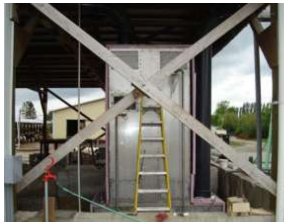
Ammonia Absorption Tower
