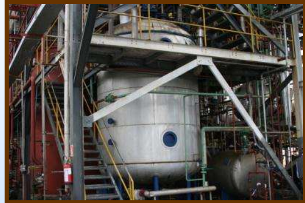
High Solid Anaerobic Digester Total Solid (TS): > 10%
