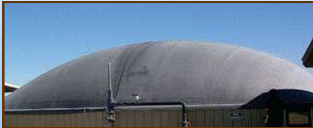
Common Anaerobic Digesters Total Solid (TS): ~5%
